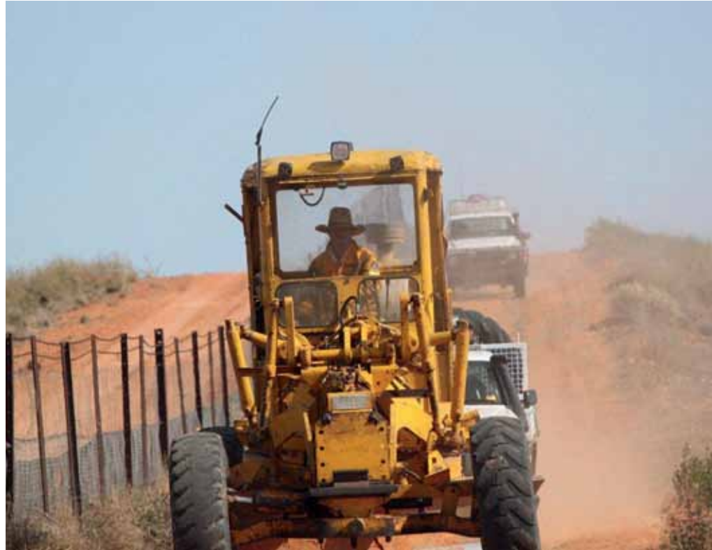
A grader working along the dog fence building containment lines on the NSW/SA border. Photo by Mark Lacy
