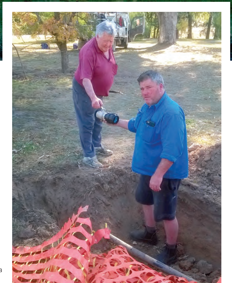
ABOVE: Steve Bugden commencing the fit-out of the sprinkler irrigation system at Billy Grace Reserve
