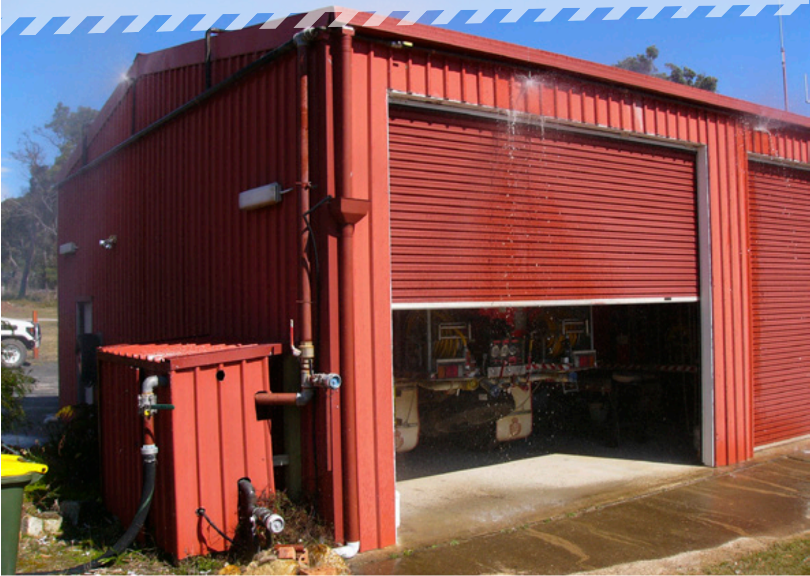
Above: The drenching system in operation at the Wonboyn brigade station. Photo by Paul Cook.
