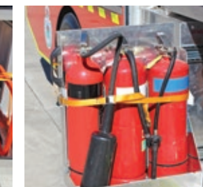
Extinguishers on slide out mechanism
